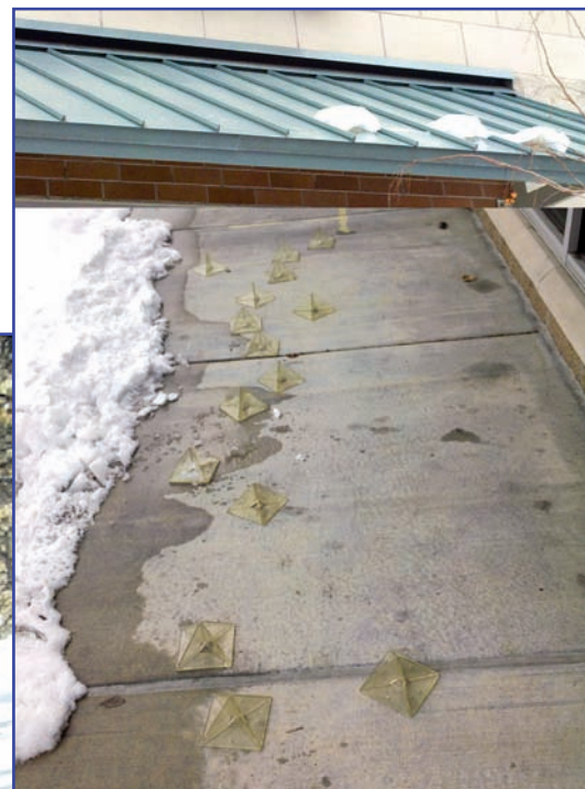
Photo 2 – These plastic snow guards fell to the ground because the adhesive did not bond properly.
