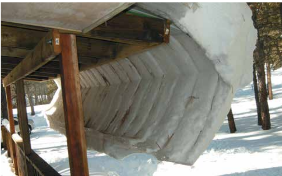
Figure 4. Snow creeping and curling over the edge of a roof.
