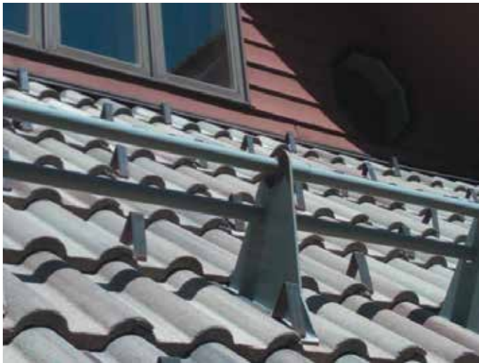
Figure 7. Water flows under snow retention devices and freezes around snow guards in the roof field.
