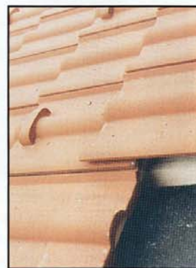
These tiles have affixed concrete snow stops. Note the vented system between deck and tile, at right.
